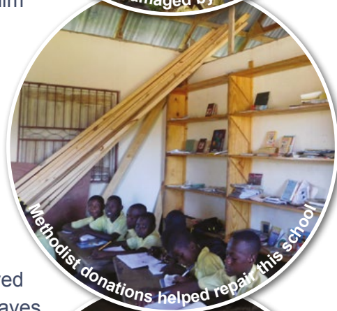
Methodist school damaged by Hurricane Matthew
